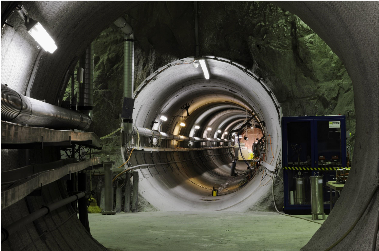
Photograph of an underground test tunnel in the Grimsel test site. (credit: Comet Photoshopping GmbH, DieterENZ.)
